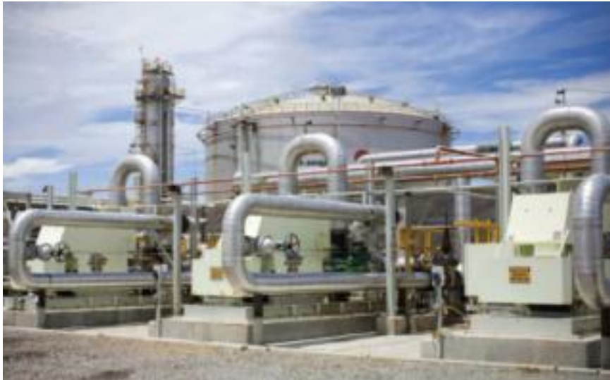
Example of a Central Processing Facility
